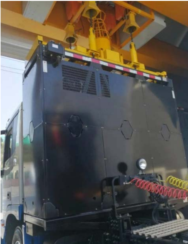
Figure 29: Battery location in this project.
